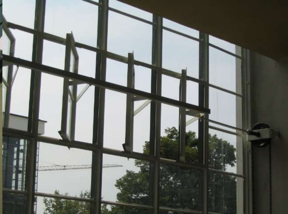
Mechanically opened windows
